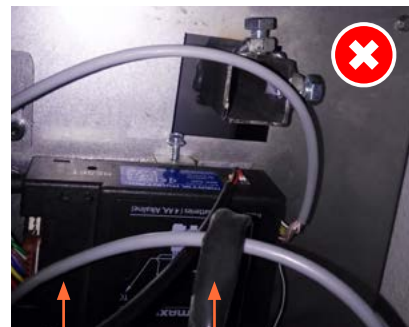
LED module cable Ignition cable
