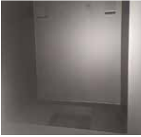
1. Clean fire chamber.
